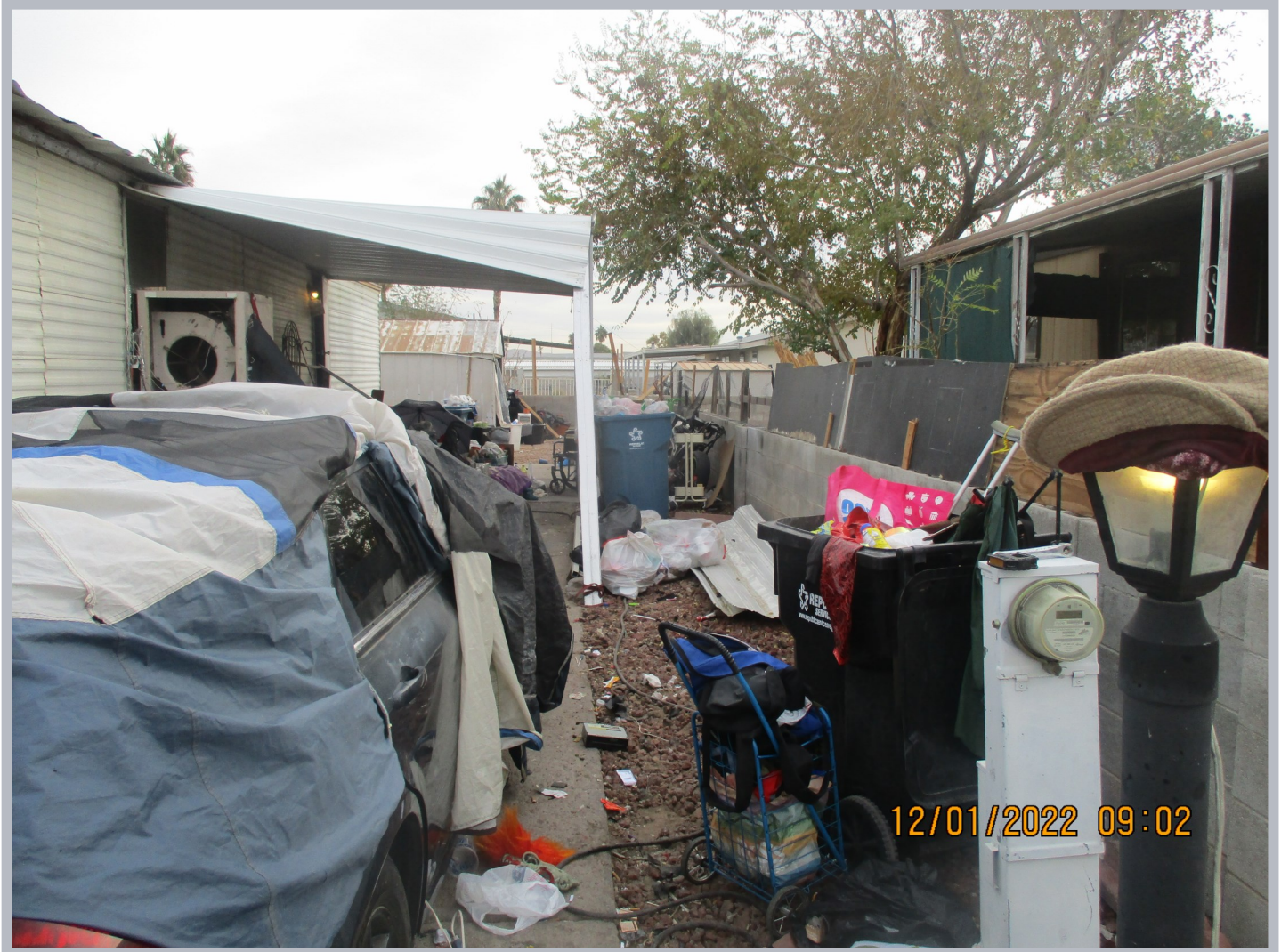
1) Outside Storage 2) Solid Waste 3) Inoperable Vehicle 4) Accessory structure as dwelling 5) Set Back violation 6) Non permitted raising of the wall. 7) restricted ingress/egress.
